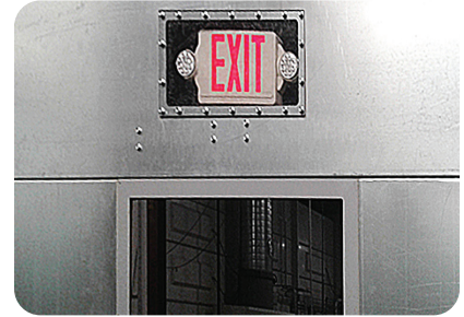
Emergency Exit Light
